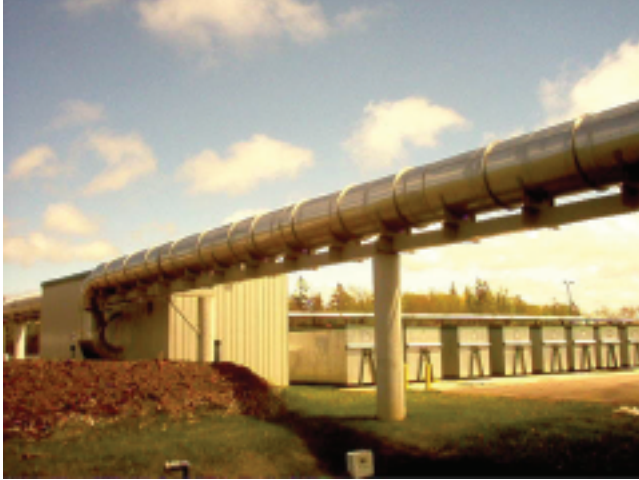
Off-gases from the composting vessels and buildings are treated in a biofiltration system.
